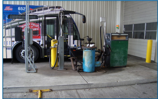
This outdated fuel pump at Southwest Division in Bridgeview is scheduled for replacement 2018.
