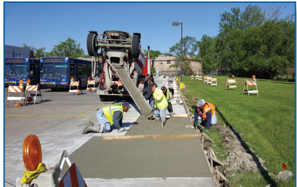
A failed culvert pipe for the storm sewer was replaced at the North Division garage.
