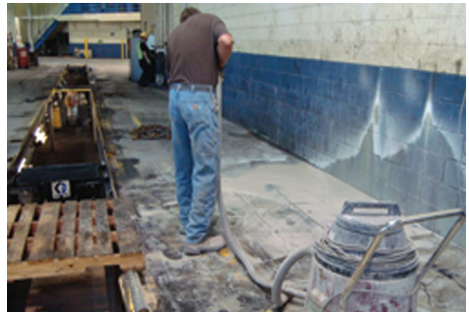
Due to aging equipment, Pace replaced a broken grease line at South Division in 2011.
