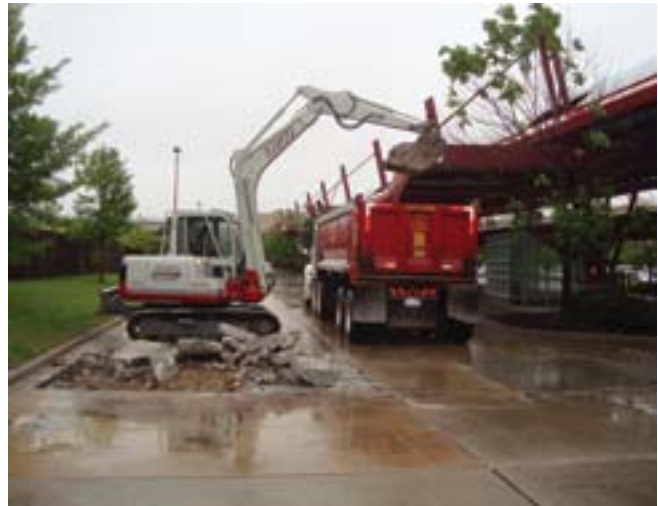
Emergency concrete repairs were necessary at the Northwest Transportation Center in Schaumburg in 2011.
