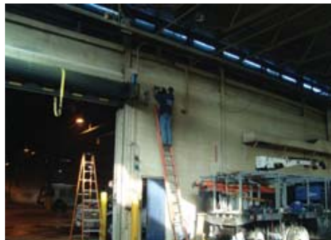
Overhead door replacements are a costly item. Pace completed a project which replaced South Division's overhead doors in 2011.
