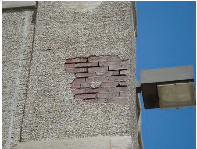
The building envelope at Heritage Division is in desperate need of replacement.
