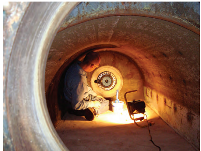
A new Burnham boiler blast tube was replaced at River Division in 2009.
