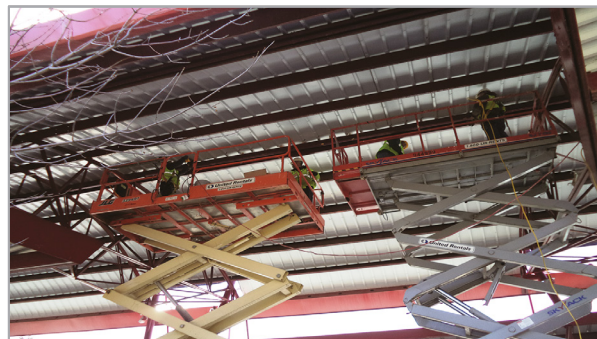
Pace completed structural steel rehab to its Northwest Transportation Center in Schaumburg in 2014.
